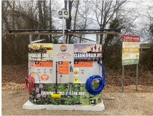
CD3 Wayside Solar watercraft cleaning station installed at Beech Creek Access on Lake Columbia, February 29, 2024.
